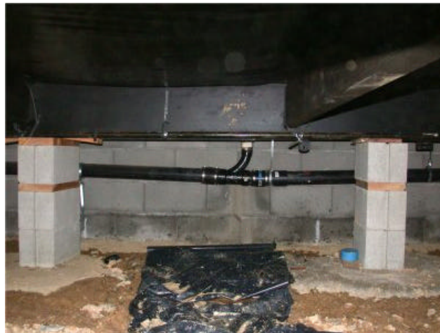
Plumbing hung at the factory can be damaged during transit or, as seen here, needs to be adjusted after the house is in place. Sagging pipes are likely to back up or crack from stress. Photo courtesy of Janis Paris.
